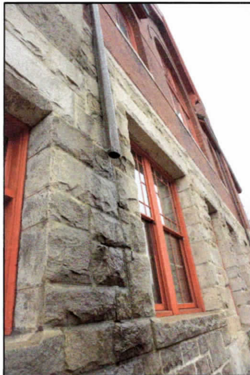
Photo 72 Missing downspout on Main Street elevation
