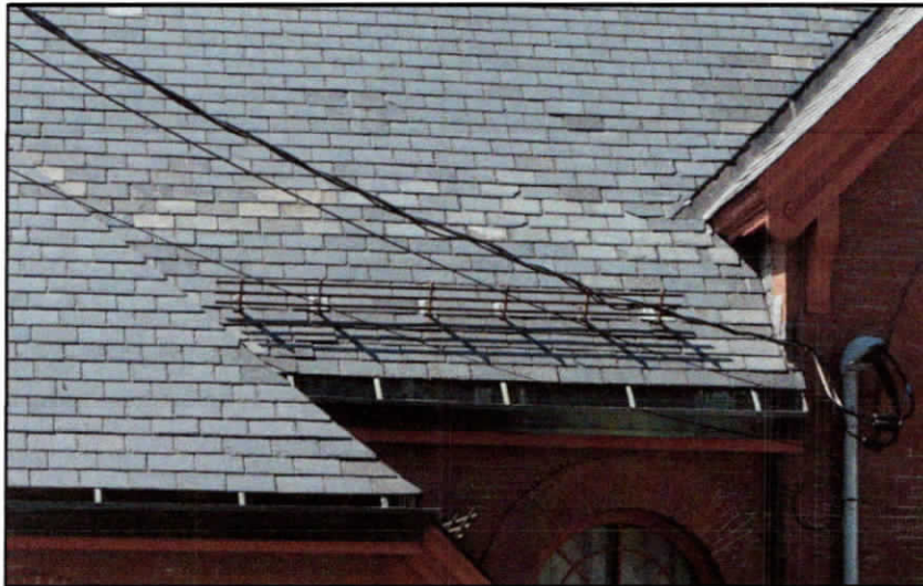
Photo 71 Broken slates on Maple Street elevation
